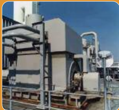
A 66,000 HP (50,000 KW) machine for a main air compressor in an air separation unit. This machine has an efficiency value of 98.82%.
