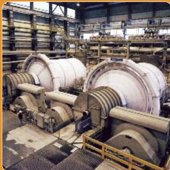
GE Quadramatic™ Drive System in a ball mill application
