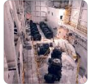
Dragline interior showing vertical and horizontal motors along with MG set.
