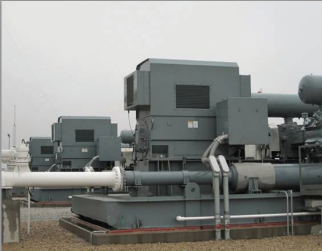
5000 HP, 900 RPM Medium Voltage Motor & Ariel Compressor Unit
