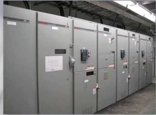
Motor Control Center Line-Up
